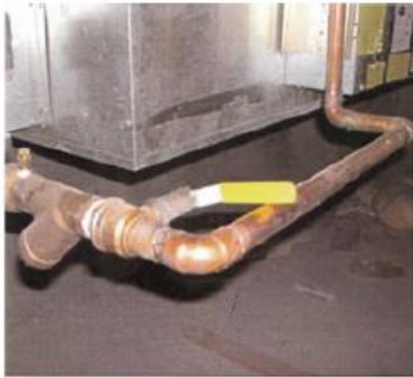
Hot water valve motion impeded by piping layout [EMC no date (a)]
