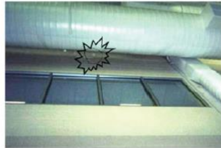
Photosensor (for daylight harvesting) shaded by duct [Deringer 2008]
