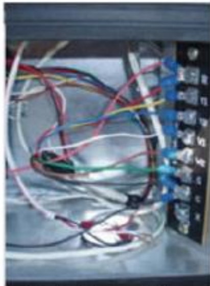
Exhaust fan hardwired in an “always on” position [Mittal and Hammond 2008]
