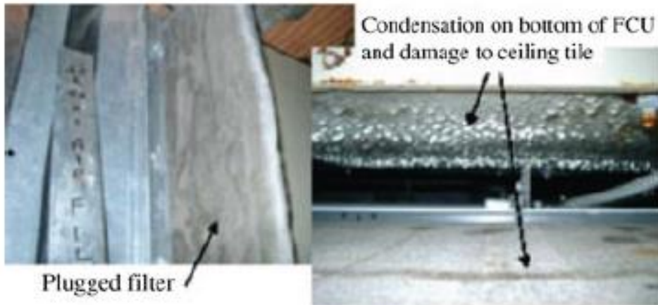
Plugged filter causing condensation on bottom of fan coil unit and damage to insulation coil resulting in poor air flow [Martha Hewett, MNCEE]
