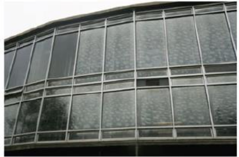
Failed window film treatment
